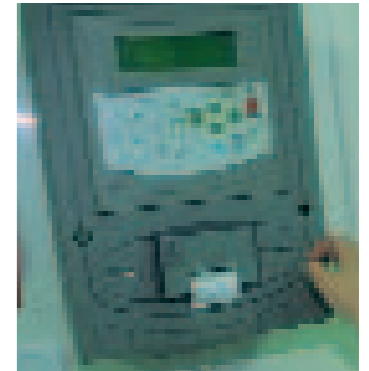
Chill room temperatures are regularly checked
